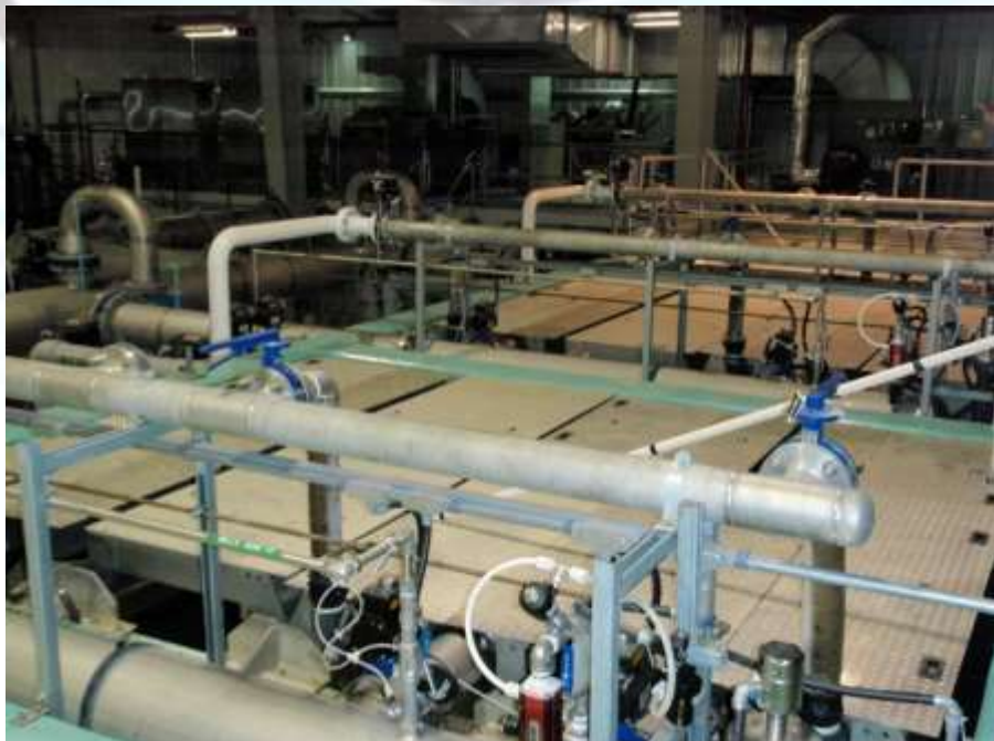
Arrow Creek Water Treatment Plant
