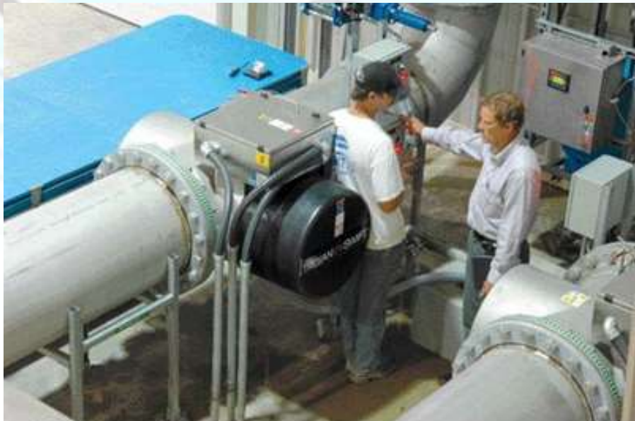
Arrow Creek Ultra Violet Disinfection Equipment
