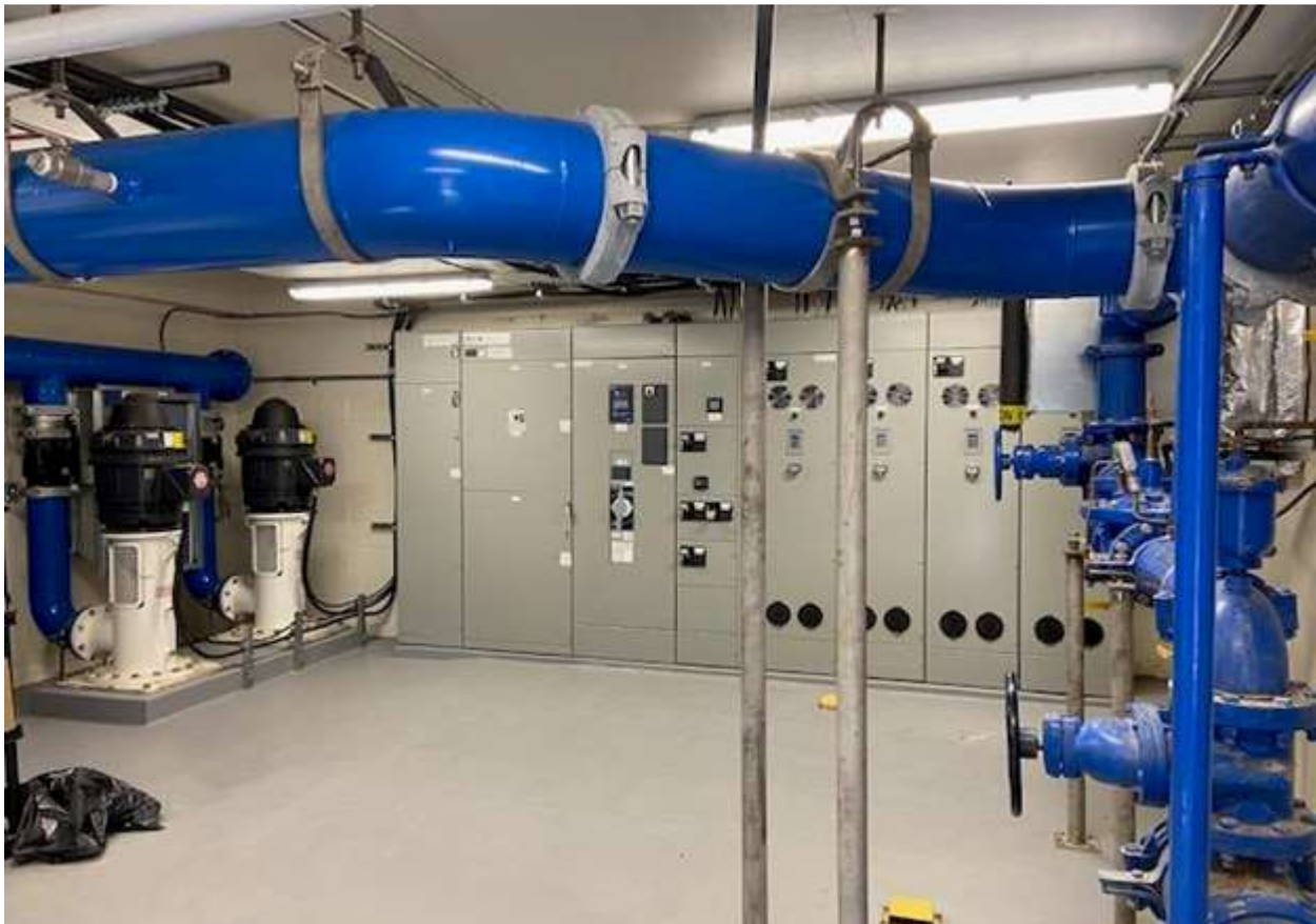
Schikurski Park Booster Pump Station
