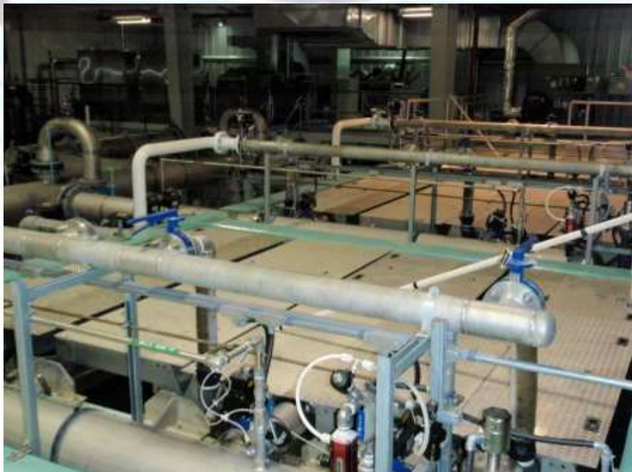
Arrow Creek Water Treatment Plant
