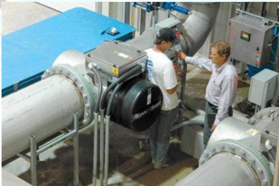
Arrow Creek Ultra-violet Disinfection Equipment
