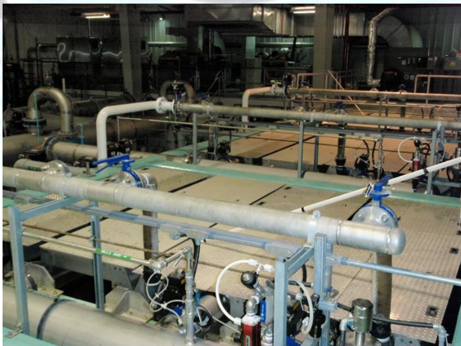
Arrow Creek Water Treatment Plant
