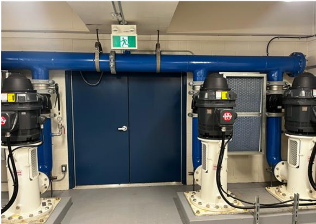
Schikurski Park Booster Station
